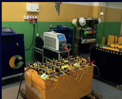
Punaha utilizes a software-controlled 'desulphation process' which can regenerate lead acid batteries to be used twice longer
